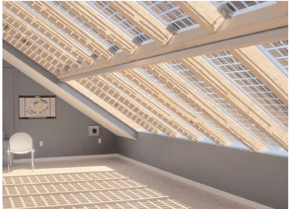
Photo 2: Attic space with BIPV roof
